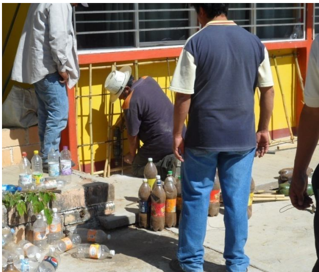
Figure 11. Construction technique implemented on classroom walls to isolate them. (Photo: J. Caballero, 2010)
